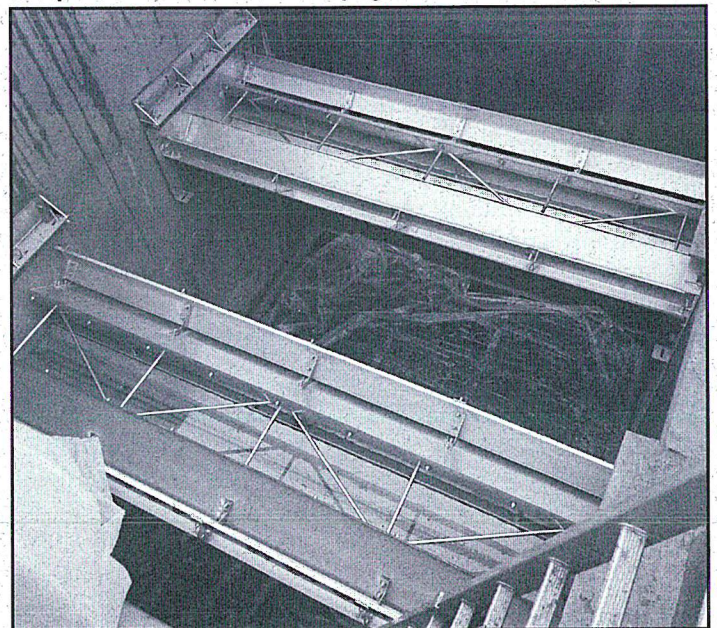
The new treatment plant has concrete gravity filters.
